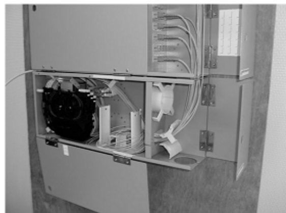
Figure 7: Optical connection box for the pilot
